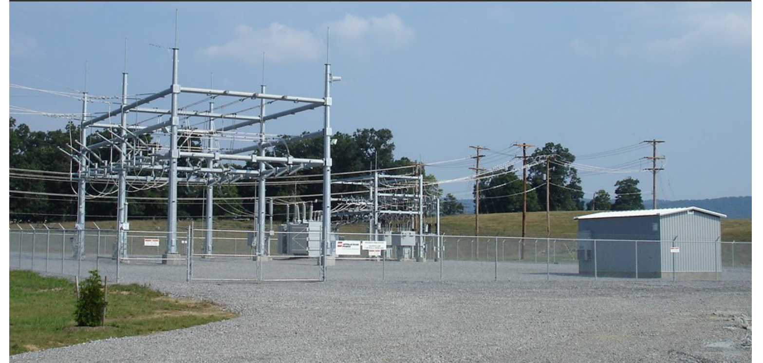
Substation shown is a general depiction of the proposed facilities for the project. It does not represent a final design.
