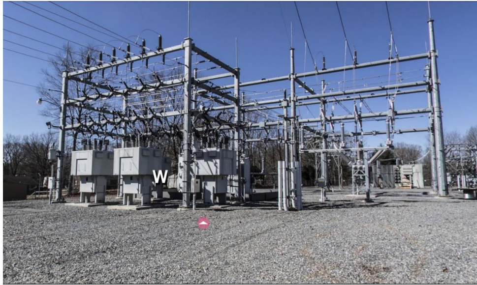
EXISTING BRUSH TAVERN SUBSTATION (VIEWING TO THE NORTHWEST)
