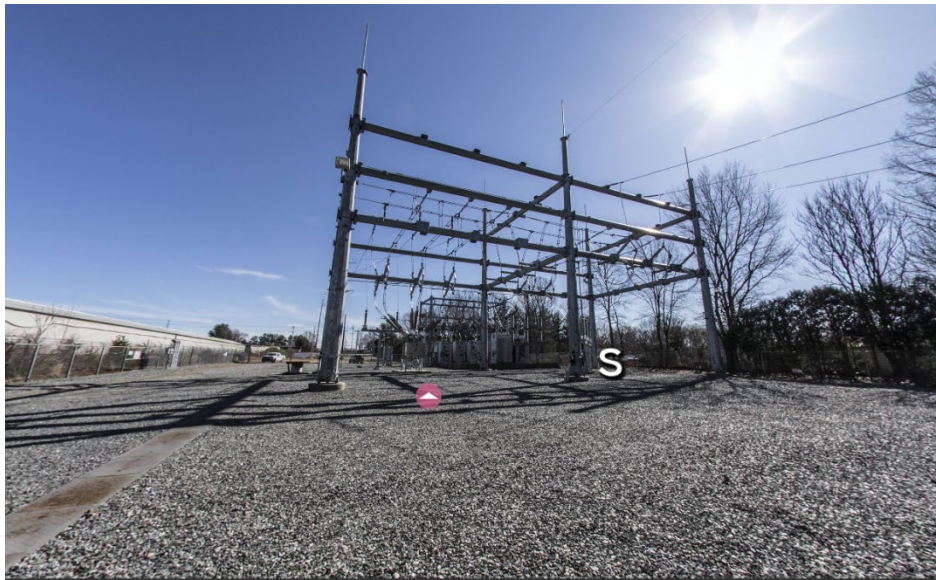
EXISTING BRUSH TAVERN SUBSTATION (VIEWING TO THE SOUTH)
