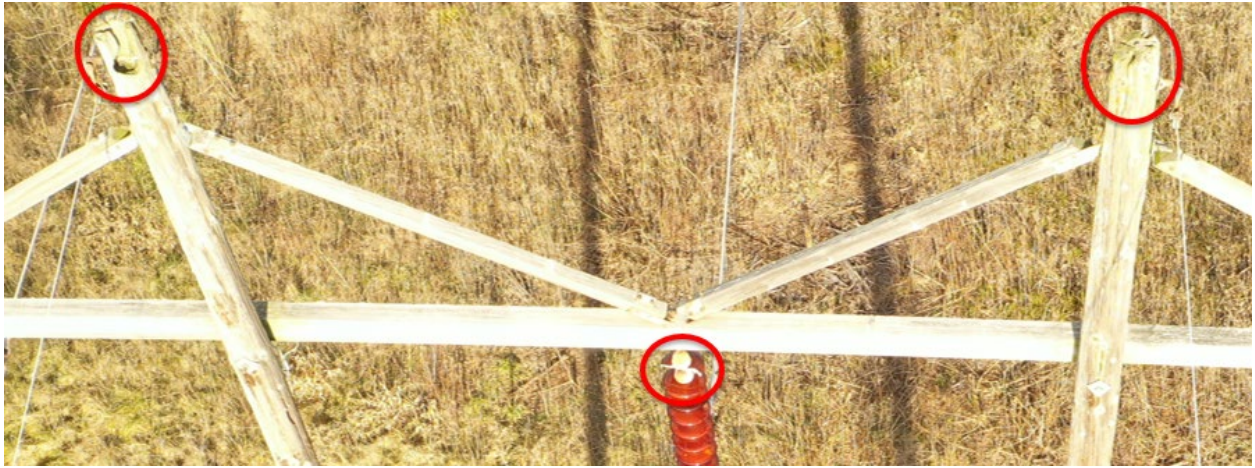
Figure 15 Structure 47: Pole Top Cavity, Broken Insulator in String, and Pole Rot Top
