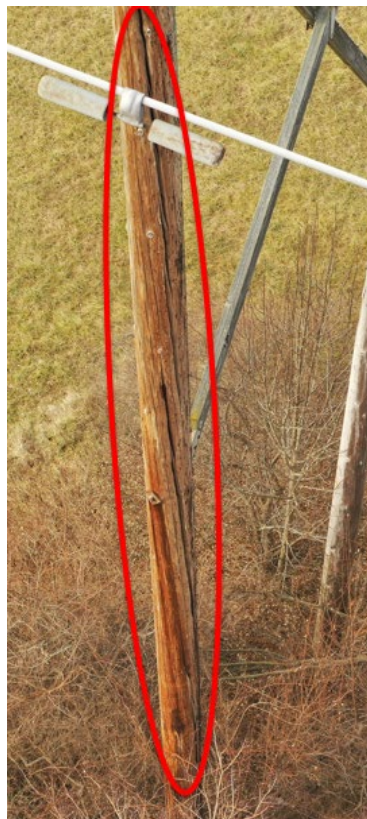
Figure 14 Structure 37: Vertical Pole Splitting from Base
