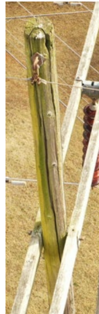
Figure 12 Structure 33: Upper Pole Splitting and Decay
