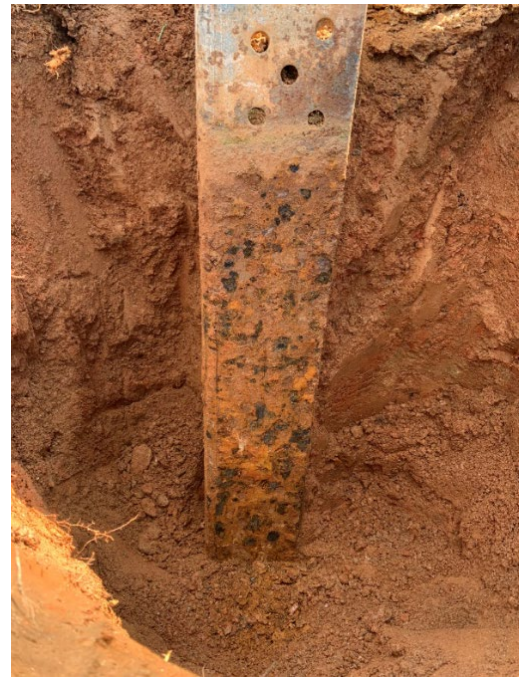
Figure 17 Structure 2: Groundline Corrosion of Steel Tower Leg
