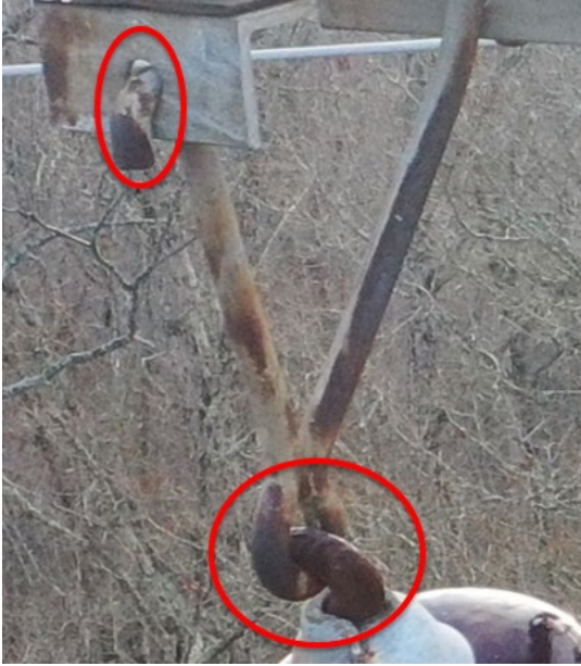
Figure 5 Structure 2: Structure Attachment Points, Corrosion of Insulator Hardware, and Degradation of Insulator Attachment Hook
