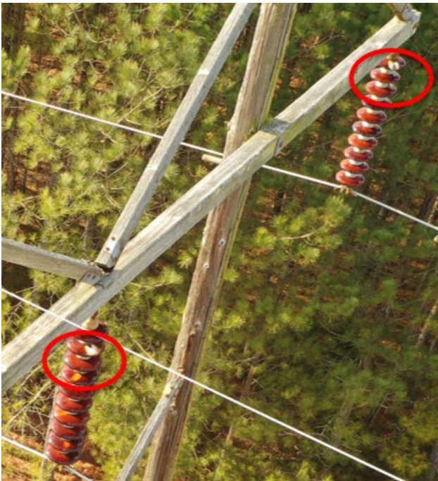
Figure 16 Structure 47: Insulators with Flashover/Arcing Damage
